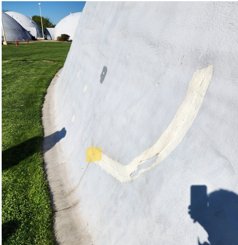
FIGURE 24: DOME B PREVIOUS EXTERIOR REPAIR WITH LOCATION OF WATER LEAK OBSERVED HIGHLIGHTED IN YELLOW
