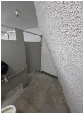
FIGURE 80: DOME CURVATURE AT MEN'S PUBLIC RESTROOM
