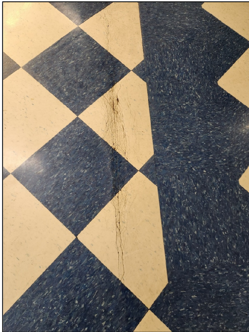
FIGURE 7: ATRIUM PERIMETER FLOORING CRACKING
