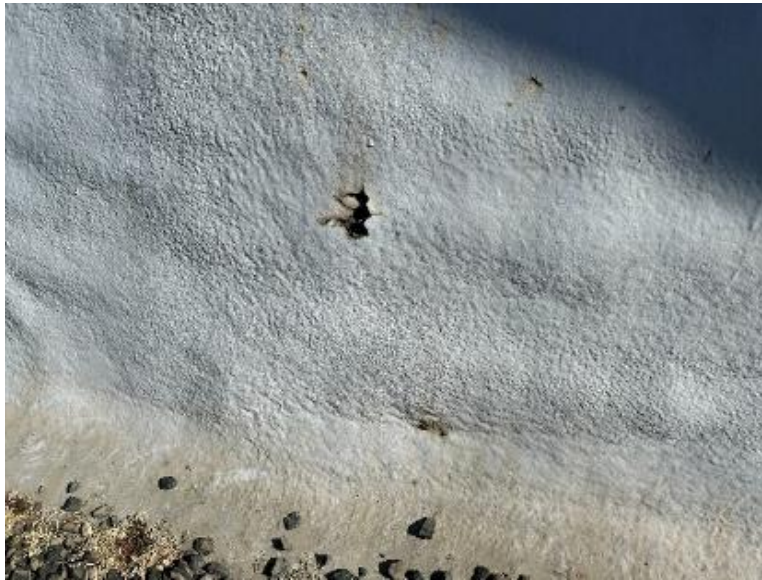
FIGURE 27: HOLE THROUGH ROOF COATING AT REPAIRED ROOF AREA ON DOME #4.
