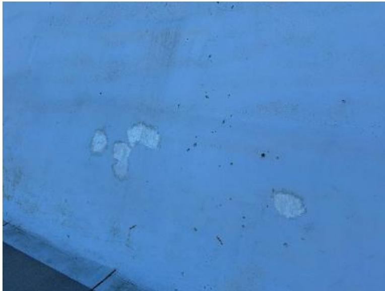
FIGURE 23: SEVERAL HOLES THROUGH THE ORIGINAL ROOF MEMBRANE WITH EVIDENCE OF PREVIOUS REPAIRS AT DOME #4.
