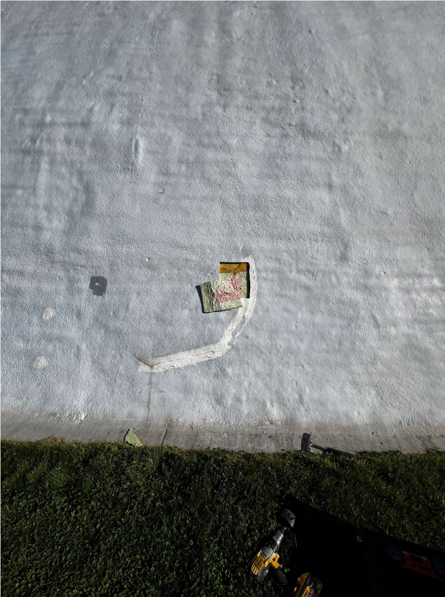
Leaking area of roofing membrane opened for coring at Dome B.
