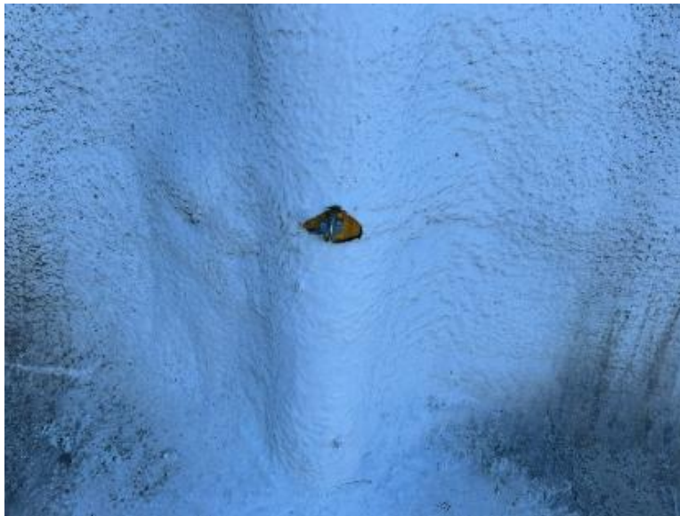
FIGURE 26: HOLE THROUGH ROOF COATING AND SPRAY FOAM AT REPAIRED ROOF AREA ON DOME #1.
