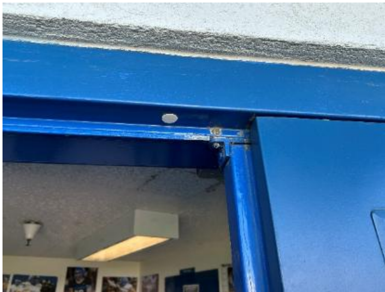
FIGURE 45: HOLLOW METAL FRAME SHOWING LACK OF THERMAL BREAK.
