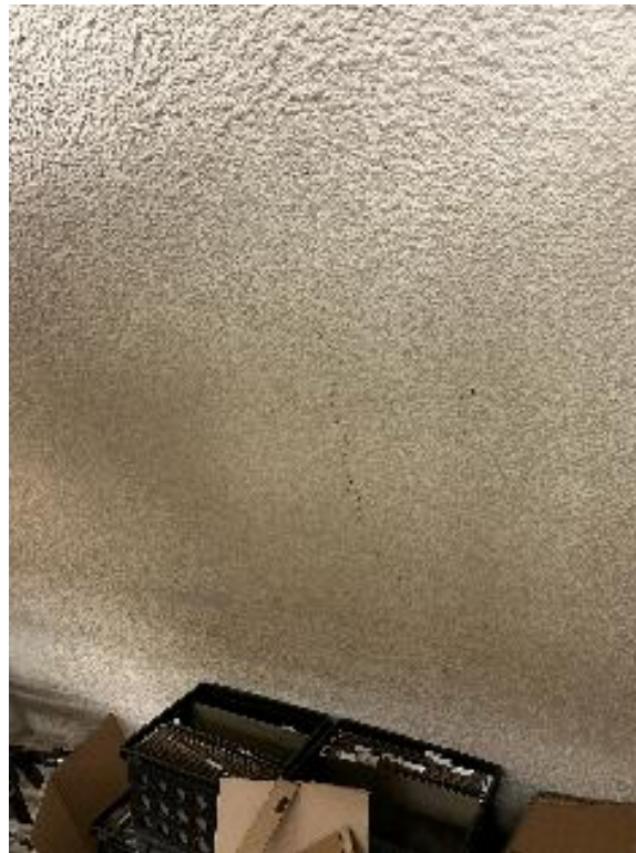
FIGURE 34: CRACK IN CONCRETE OBSERVED IN CLASSROOM 108.
