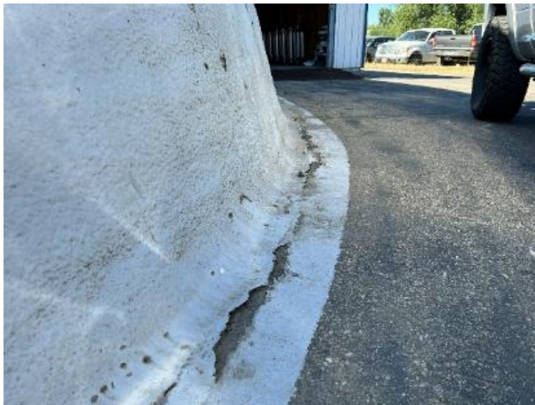
FIGURE 168: ROOF COATING AT REPAIRED ROOF AREA ON DOME #5 DEBONDED FROM HORIZONTAL CONCRETE.
