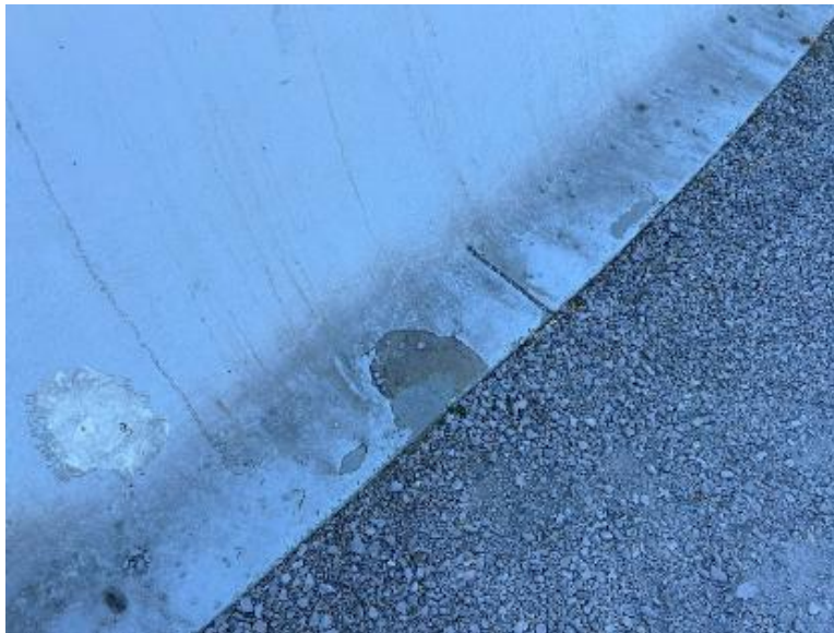
FIGURE 20: ORIGINAL ROOF MEMBRANE AT DOME #1 DEBONDING FROM HORIZONTAL CONCRETE.
