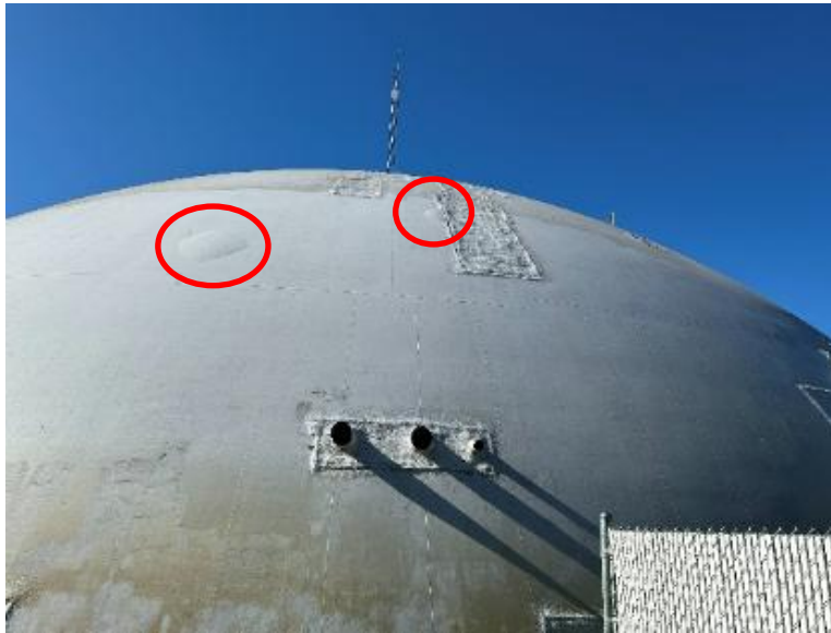
FIGURE 157: BUBBLES IN ROOF MEMBRANE AT DOME #1.
