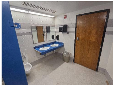
FIGURE 50: MISSING TOILET PARTITION
