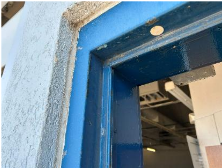
FIGURE 47: PAINTED GASKETS AT HOLLOW METAL DOOR, WHICH LIMITS THE ABILITY FOR THE GASKETS TO SEAL.
