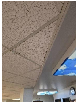
FIGURE 42: EXAMPLE OF DAMAGED TILE
