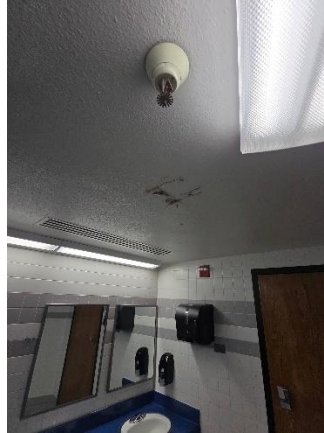
FIGURE 66: FIRE SPRINKLER FIXTURE
