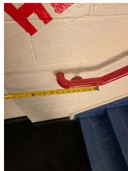
FIGURE 95: HANDRAIL EXTENSIONS NOT EXTENDING REQUIRED AMOUNT
