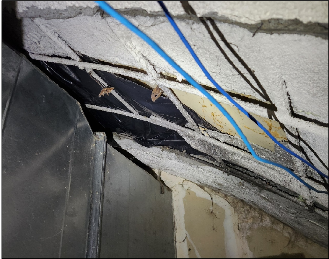
FIGURE 17: DOME B MECH SPACE EXPOSED REINFORCEMENT – LOCATION 2
