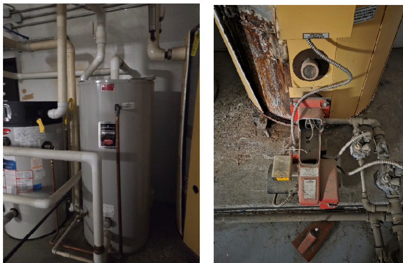
FIGURE 8: DOMESTIC WATER HEATER EQUIPMENT
