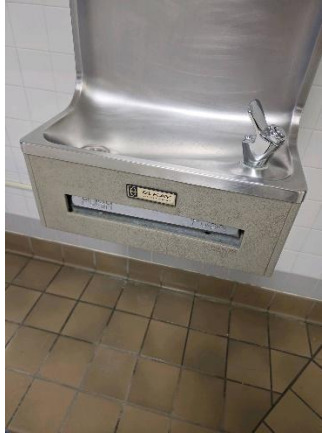
FIGURE 54: DAMAGED DRINKING FOUNTAINS
