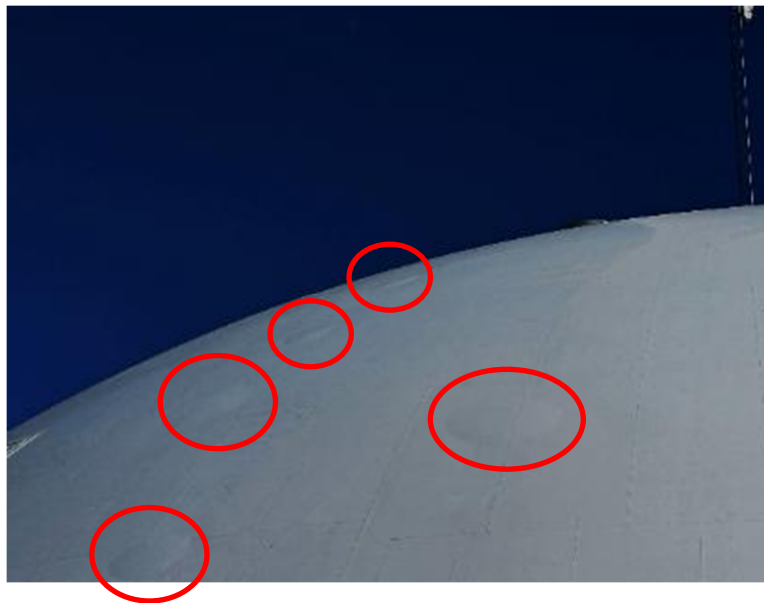
FIGURE 146: BUBBLES IN ROOF MEMBRANE AT DOME #1.
