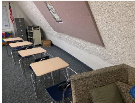
FIGURE 76: DOME CURVATURE IN A CLASSROOM
