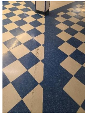
FIGURE 33: CRACKED VCT AT THE ATRIUM
