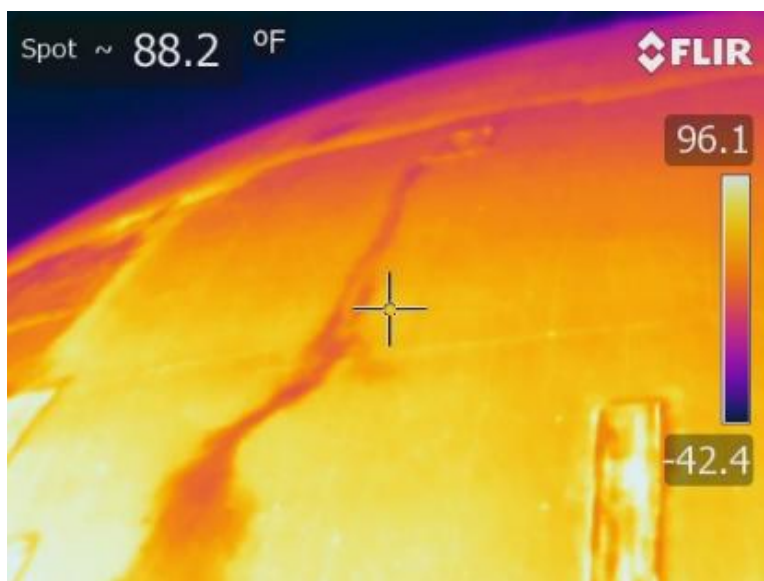
FIGURE 11: IR IMAGE OF SAME AREA AS FIGURE 10 SHOWING TEMPERATURE ANOMALIES RUNNING DOWN FROM BOTTOM CORNER OF PATCHED AREA.
