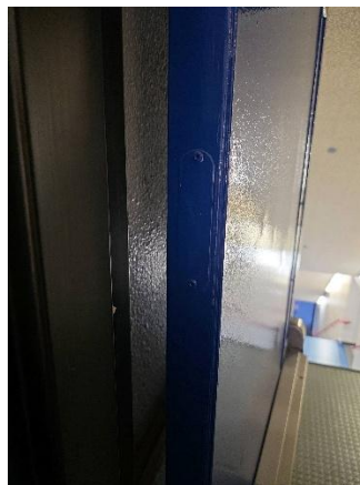
FIGURE 65: FIRE DOOR RATING TAG
