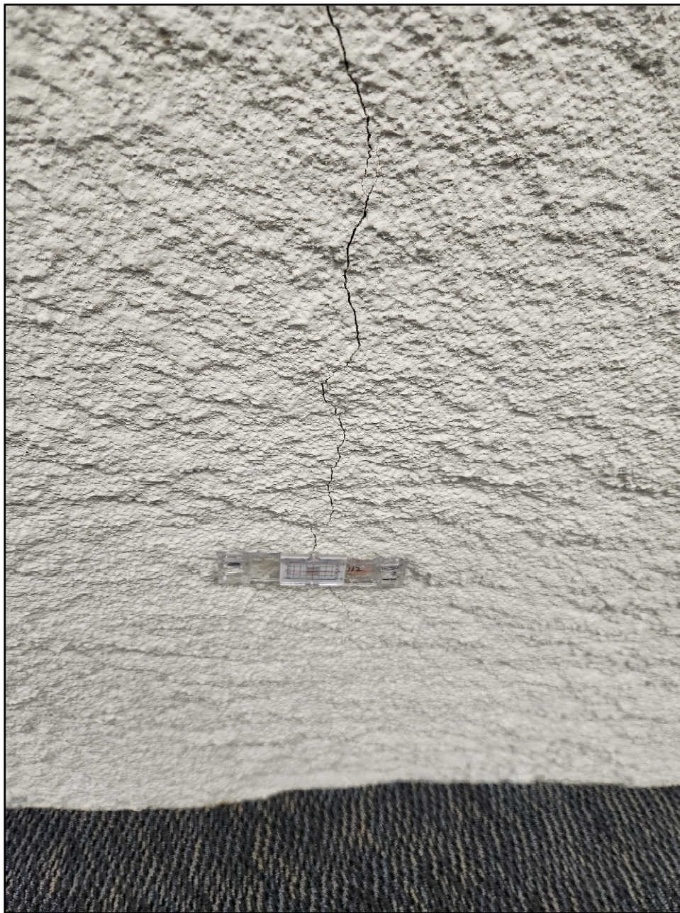
FIGURE 12: DOME A CRACK WITH STRAIN GAUGE PER ATLAS (CLASSROOM)
