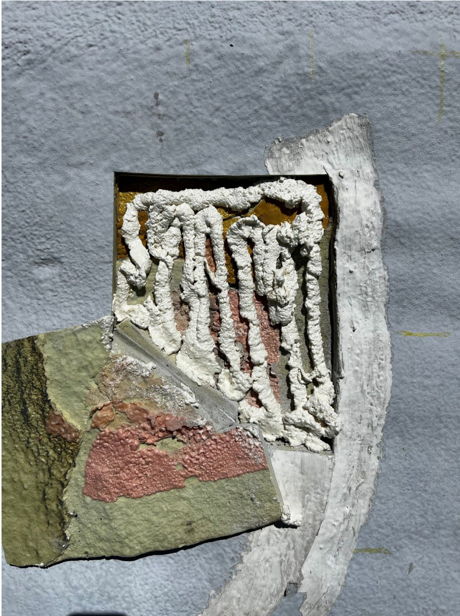
Spray urethane foam was used to re-adhere the membrane.
