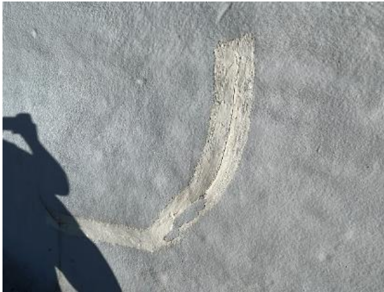
FIGURE 28: SPLIT IN ROOF COATING AND FOAM BEFORE REMOVAL WITH EVIDENCE OF PREVIOUS REPAIR.
