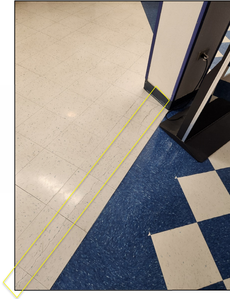
FIGURE 9: ATRIUM PERIMETER FLOORING CRACKING
