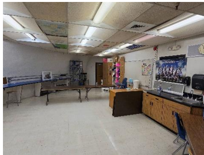
FIGURE 41: AGED TILE IN CLASSROOM
