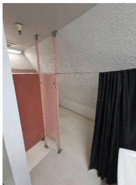
FIGURE 53: MISSING STAFF PARTITION
