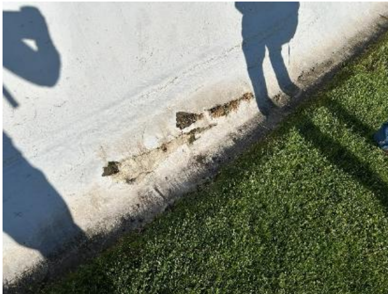
FIGURE 21: ROOF COATING AT REPAIRED ROOF AREA ON DOME #2 DEBONDED FROM HORIZONTAL CONCRETE, ALLOWING ORGANIC GROWTH TO OCCUR.
