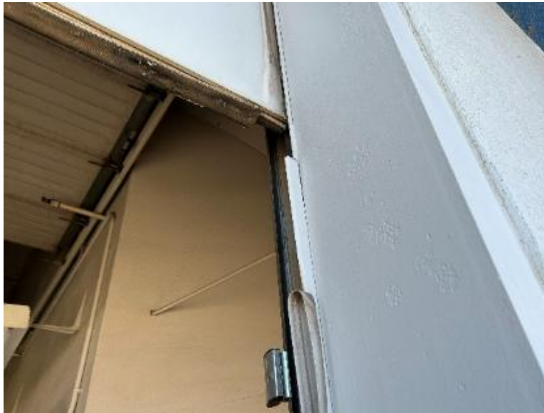
FIGURE 50: DAMAGED/MISSING GASKETS AT OVERHEAD COILING DOORS.
