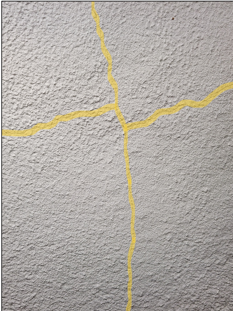
FIGURE 14: DOME B CRACKS IN THE MUSIC ROOM STORAGE AREA WITH CRACK LOCATIONS HIGHLIGHTED IN YELLOW
