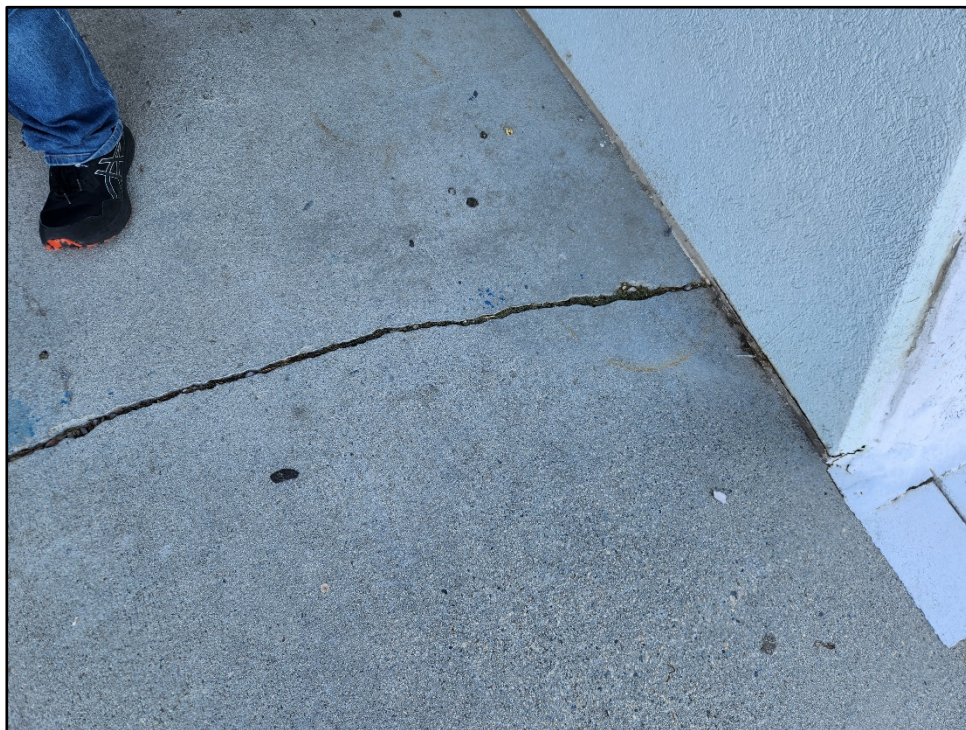
FIGURE 19: SLAB-ON-GRADE CRACKING AT MUSIC ROOM EXTERIOR
