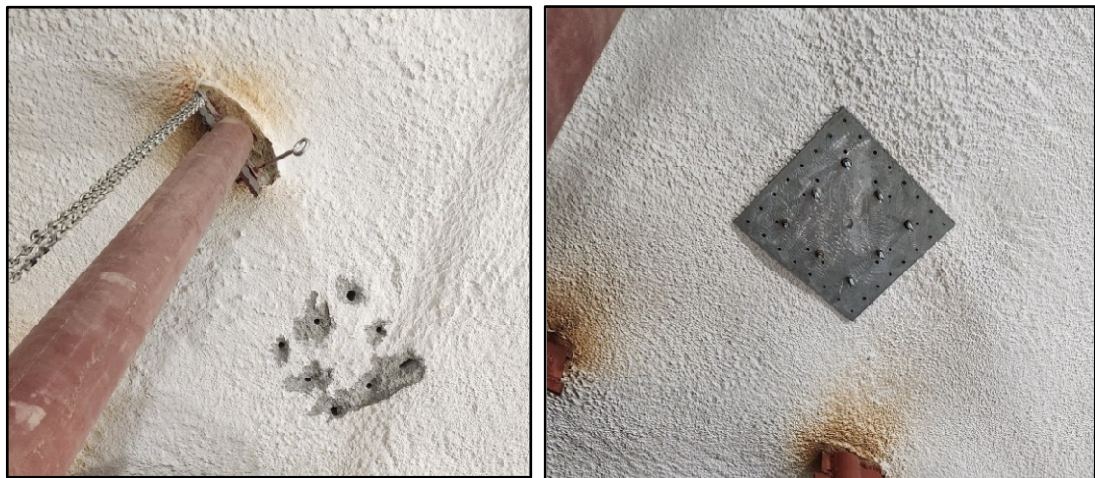
FIGURE 2: PREVIOUS ATTACHMENTS FOR ROOF TIE-OFF ANCHORS
