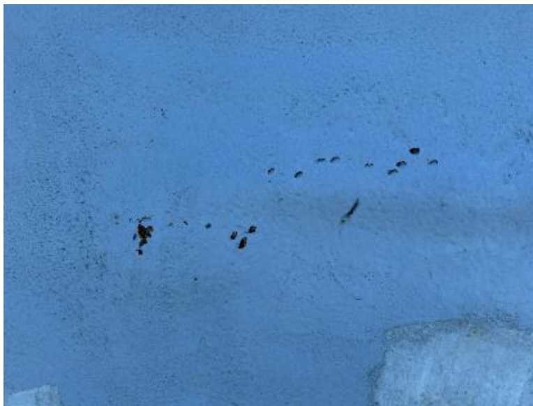
FIGURE 24: SEVERAL HOLES THROUGH THE REPAIRED ROOF AREA AT DOME #2.
