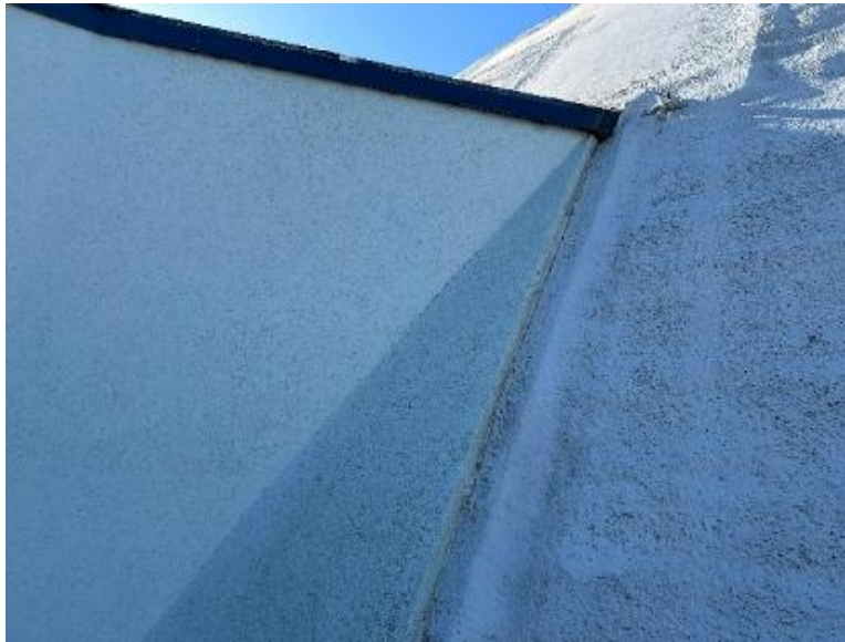
FIGURE 48: SKYWARD FACING EIFS CLADDING INTERFACING DIRECTLY WITH REPAIRED ROOF AREA.
