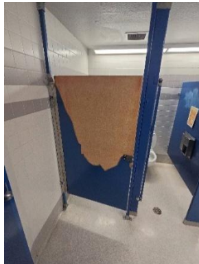
FIGURE 49: DAMAGED TOILET PARTITION
