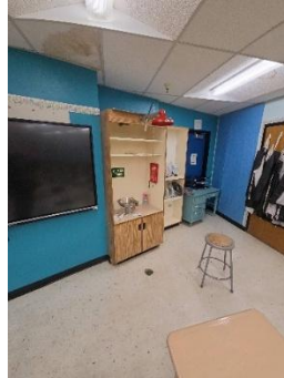
FIGURE 40: STAINED CEILING TILES IN LAB
