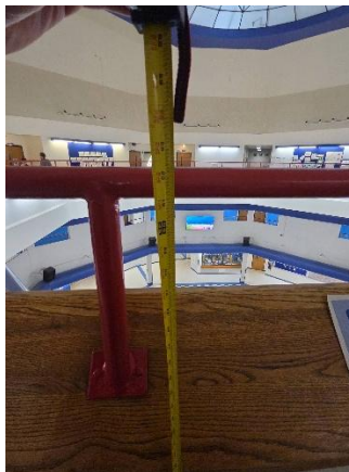
FIGURE 92: ATRIUM GUARDRAIL HEIGHT
