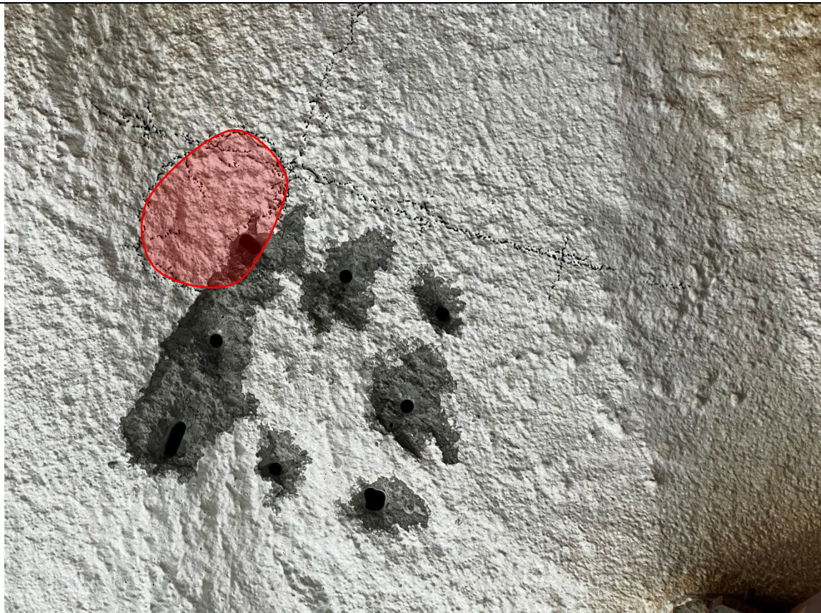
Location 6 clockwise from entry. Eight holes drilled for roof anchor. Small delamination at hole. Remainder of concrete was sound.
