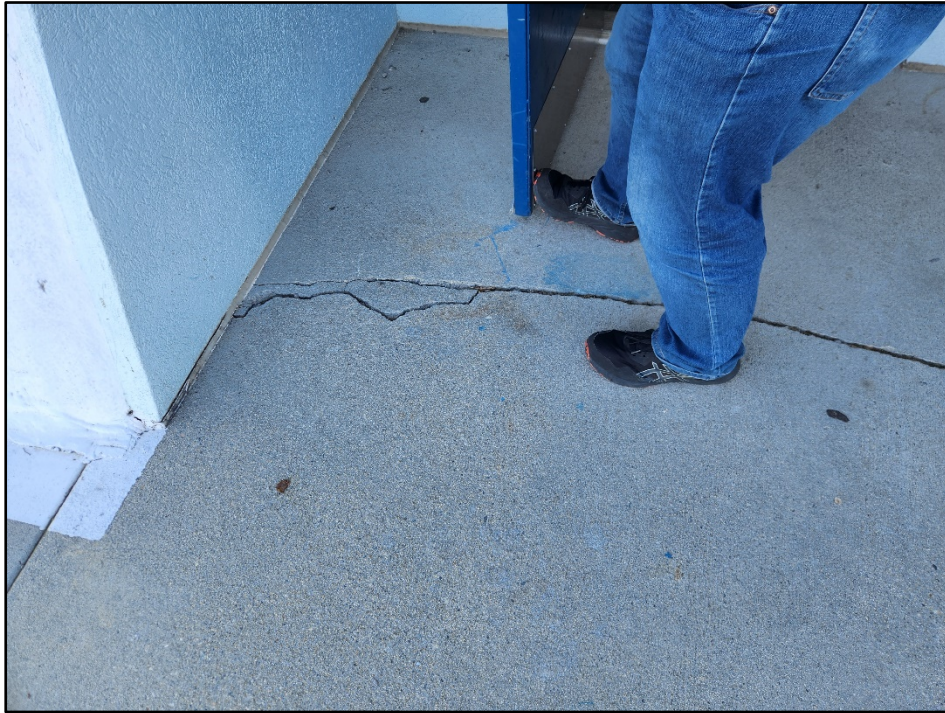
FIGURE 18: SLAB-ON-GRADE CRACKING AT MUSIC ROOM EXTERIOR
