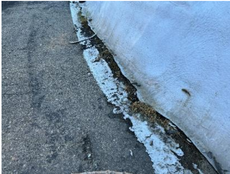
FIGURE 179: ROOF COATING AT REPAIRED ROOF AREA ON DOME #4 DEBONDED FROM HORIZONTAL CONCRETE, ALLOWING ORGANIC GROWTH TO OCCUR.
