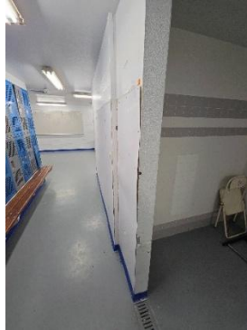
FIGURE 51: DAMMAGED WALL PROTECTION
