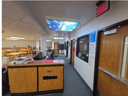
FIGURE 25: COVERINGS OVER LIGHTS IN THE LIBRARY
