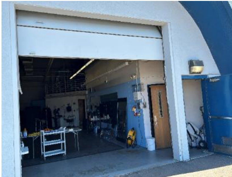
FIGURE 41: TYPICAL OVERHEAD COILING DOOR AT DOME #5.
