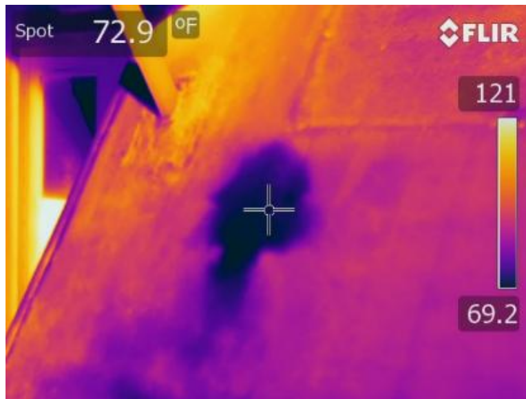
FIGURE 8: CLOSE UP OF BOTTOM LEFT CORNER OF PATCHED ROOF AREA ON DOME #1 SHOWING TEMPERATURE ANOMALY.
