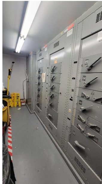
Figure 1: Existing switchboard M
