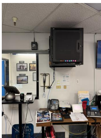
Figure 4: Wall Mtd. IT Rack in Administration Office
