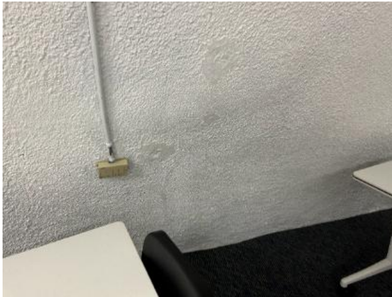
FIGURE 35: CRACKS IN CONCRETE THAT HAD RECENTLY BEEN PAINTED OVER, ROOM 110.
