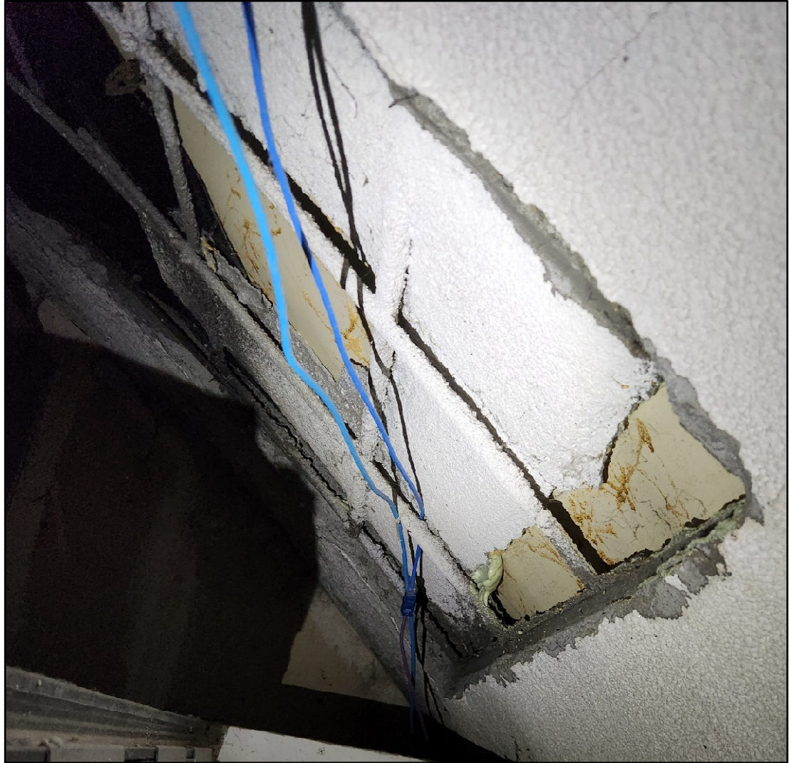
FIGURE 16: DOME B MECH SPACE EXPOSED REINFORCEMENT – LOCATION 2
