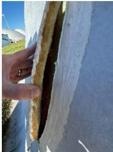
FIGURE 29: SPLIT BETWEEN LAYERS OF FOAM INSULATION.
