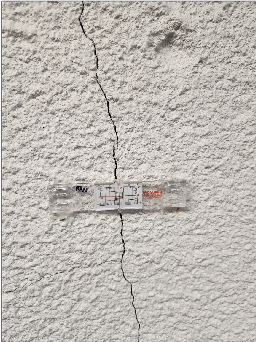
FIGURE 13: DOME B CRACK WITH STRAIN GAUGE PER ATLAS (FAN ROOM)
