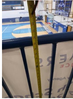
FIGURE 93: GYM GUARDRAIL HEIGHT
