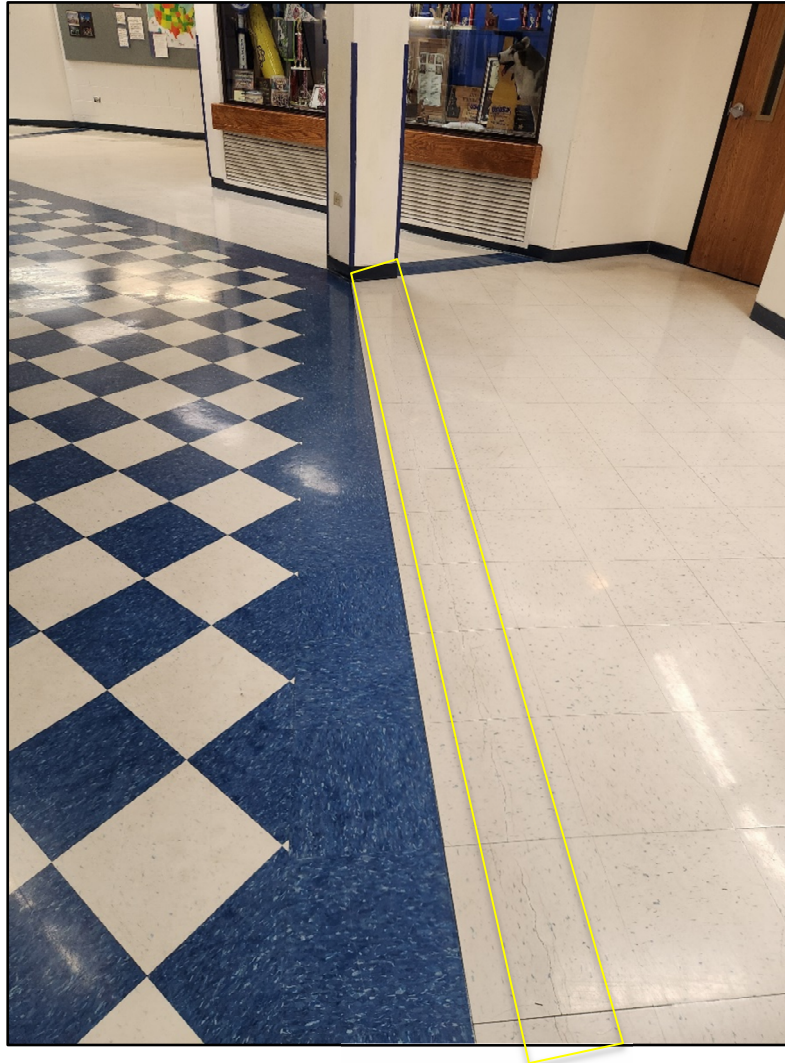
FIGURE 10: ATRIUM PERIMETER FLOORING CRACKING
