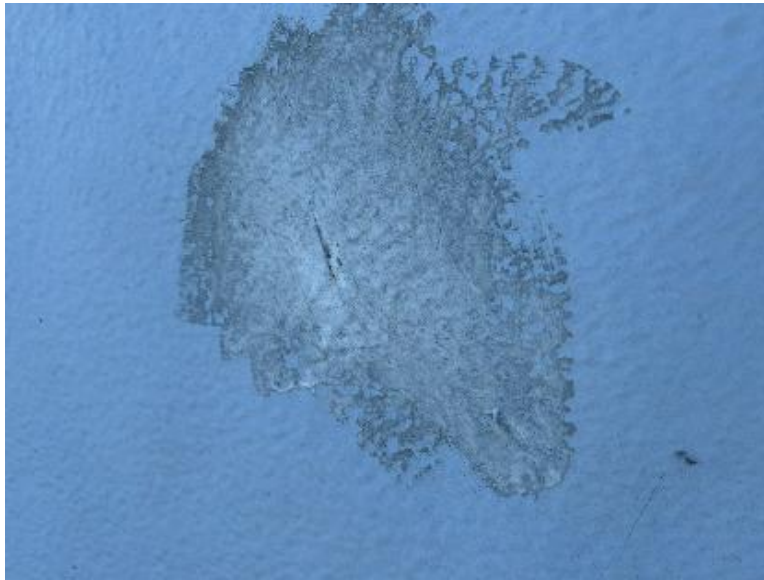
FIGURE 25: SPLIT IN ROOF MEMBRANE AT DOME #1 WITH EVIDENCE OF PREVIOUS REPAIR THAT HAS SINCE FAILED.
