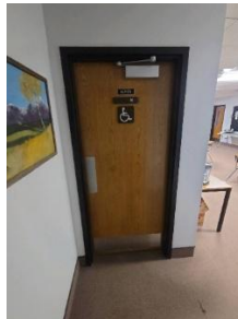
FIGURE 72: ADA DOOR CLEARNACE ISSUE
