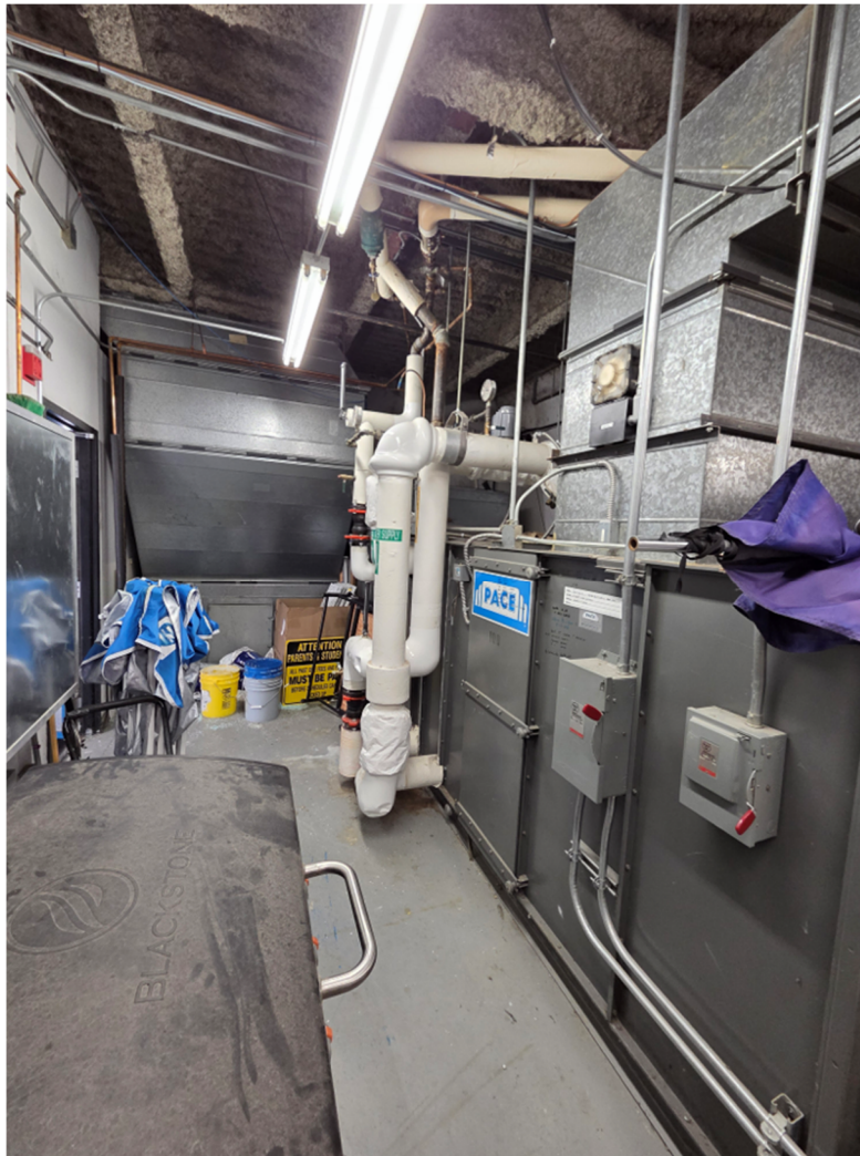
FIGURE 1: CLASSROOM LEVEL 1 AIR HANDLER
