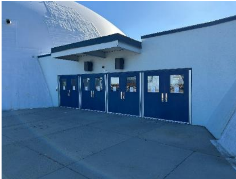
FIGURE 39: ENTRANCES AT CORRIDOR BETWEEN DOMES #1 AND #2. NOTE THAT CANOPY DOES NOT COVER ALL DOORS.
