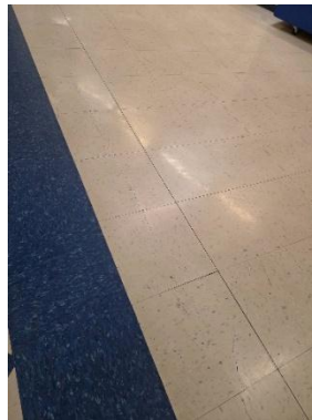
FIGURE 36: GAP IN VCT
