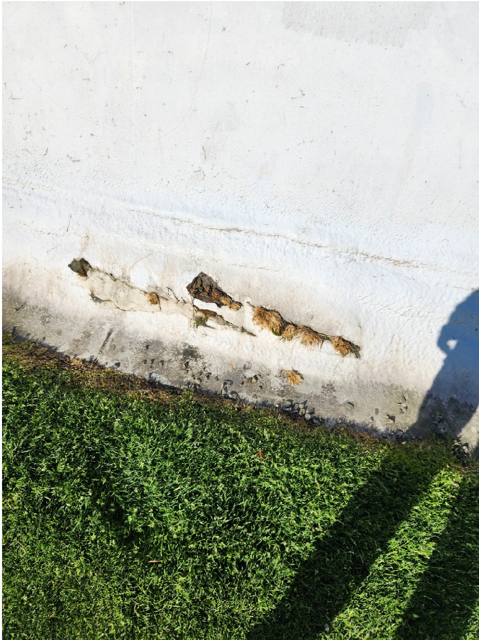
FIGURE 25: AREA OF DAMAGED EXTERIOR WITH VEGETATION GROWTH
