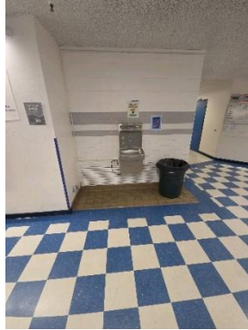
FIGURE 32: TILE AT DRINKING FOUNTAINS
