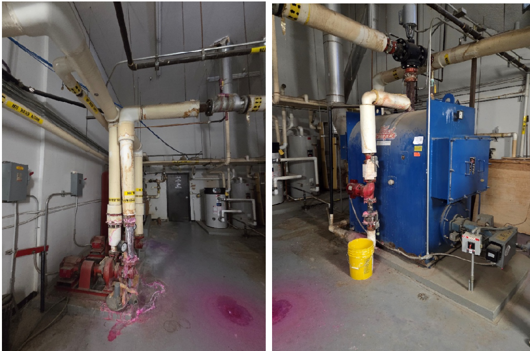
FIGURE 4: BOILER ROOM EQUIPMENT
