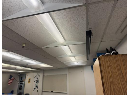
Figure 2: Classroom lighting with integral ceiling tiles
