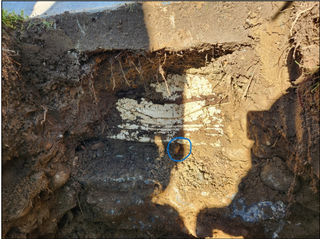
FIGURE 23: DOME “B” FOUNDATIONS AT EAST SIDE OF THE DOME WITH EXPOSED BAR CIRCLED IN BLUE
