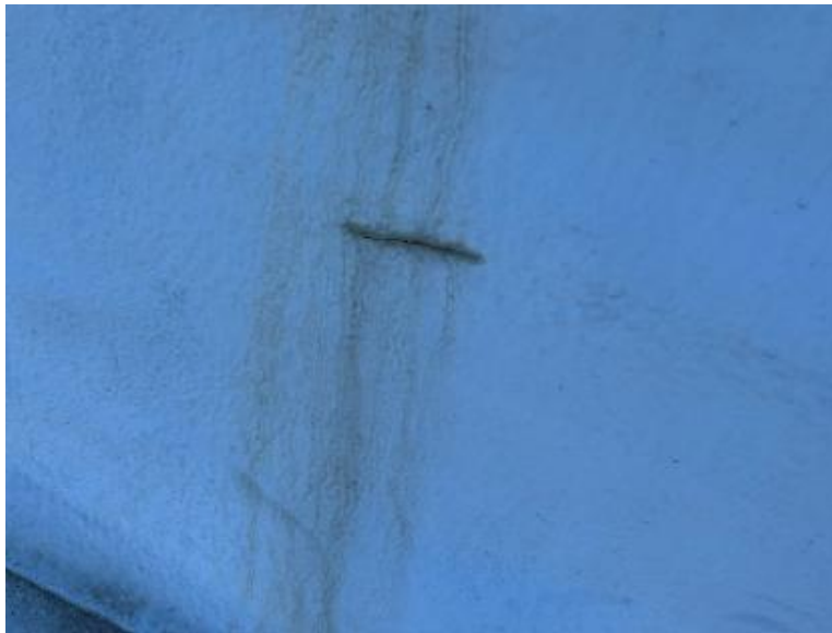
FIGURE 22: SPLIT IN ROOF COATING AT REPAIRED ROOF AREA ON DOME #4.
