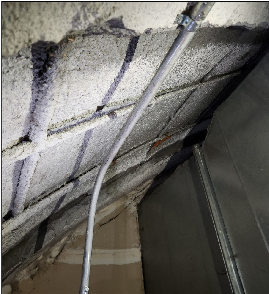
FIGURE 15: DOME B MECH SPACE EXPOSED REINFORCEMENT – LOCATION 1
