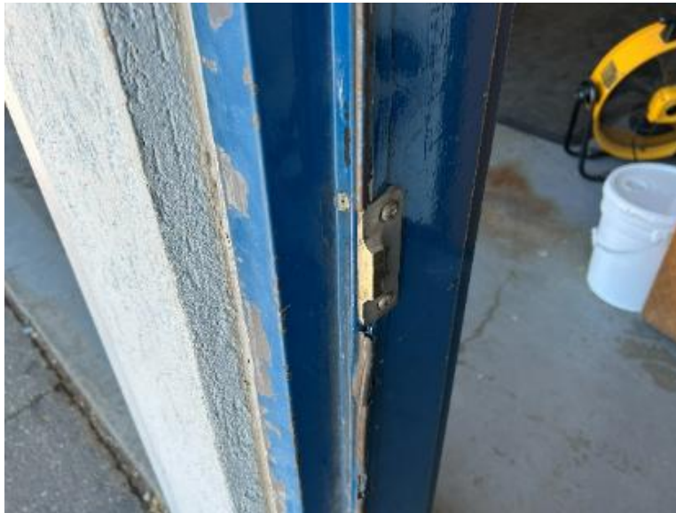
FIGURE 46: DAMAGED GASKETS AT HOLLOW METAL DOOR.
