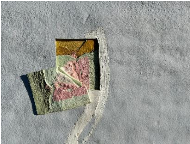
FIGURE 30: OUTER LAYER OF FOAM REMOVED, REVEALING EVIDENCE OF PREVIOUS REPAIR WITH ADDED SPRAY FOAM.
