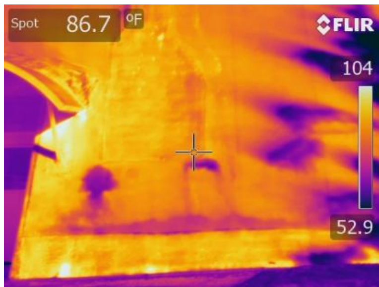
FIGURE 7: IR IMAGE OF SAME AREA AS FIGURE 6 SHOWING TEMPERATURE ANOMALIES AT LOWER CORNERS OF PATCHED AREA.
