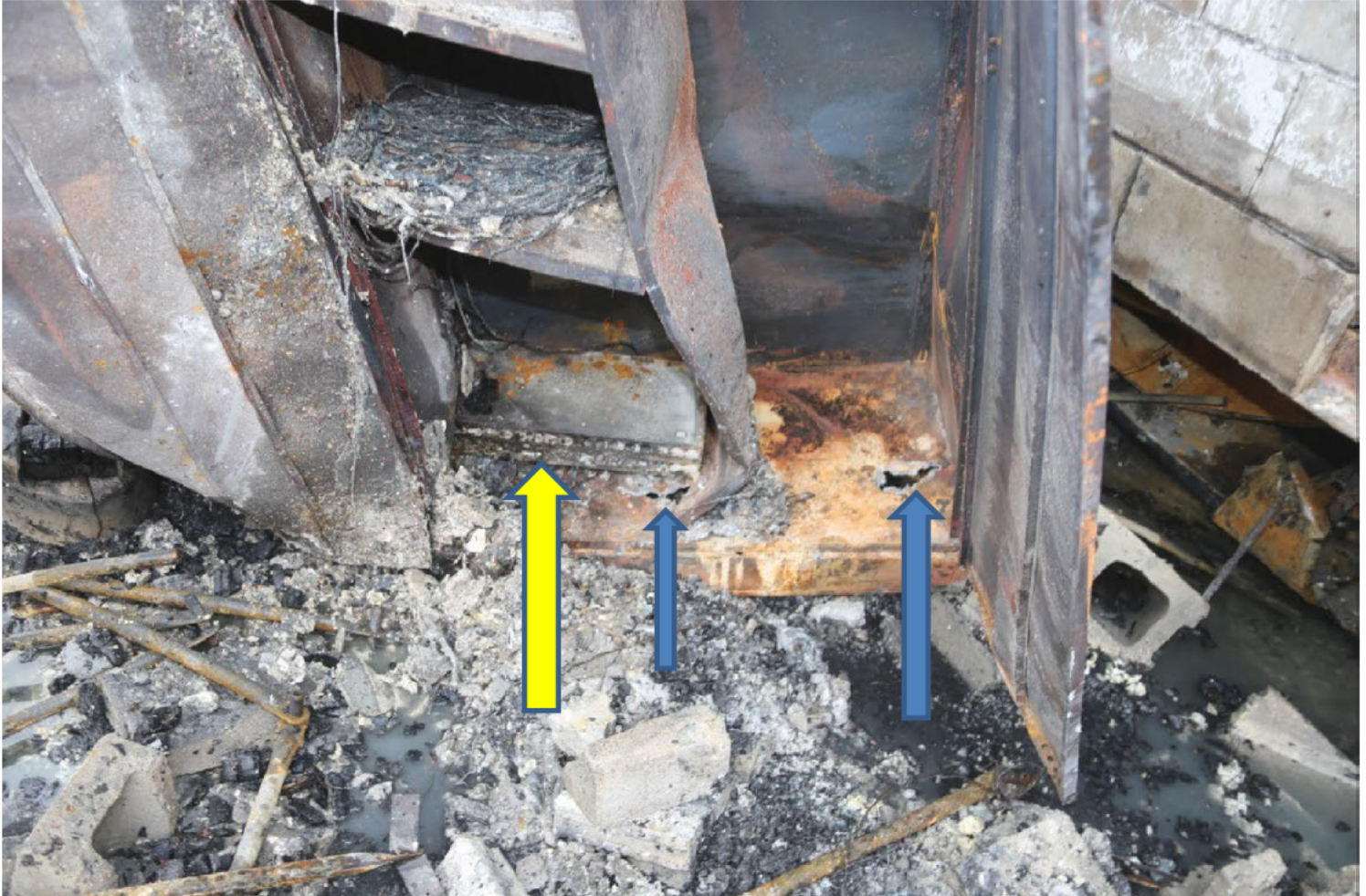
Yellow arrow showing equipment located in the cabinet on the northside of the stage area. Blue arrows show arcing inside the cabinet. Picture is from file IMG_0360.CR2. A copy of this image is included in the addenda/held in the case file.
