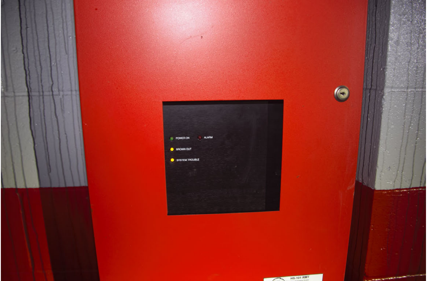
Main Alarm Panel showing Brown Out system trouble. Picture is from file IMG_0197.CR2. A copy of this image is included in the addenda/held in the case file.
